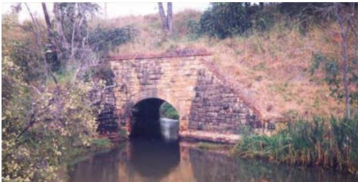
Stone railway culvert at Wooroloo, October / November 1995 (Source: Bruce Callow and Associates Pty Ltd)
