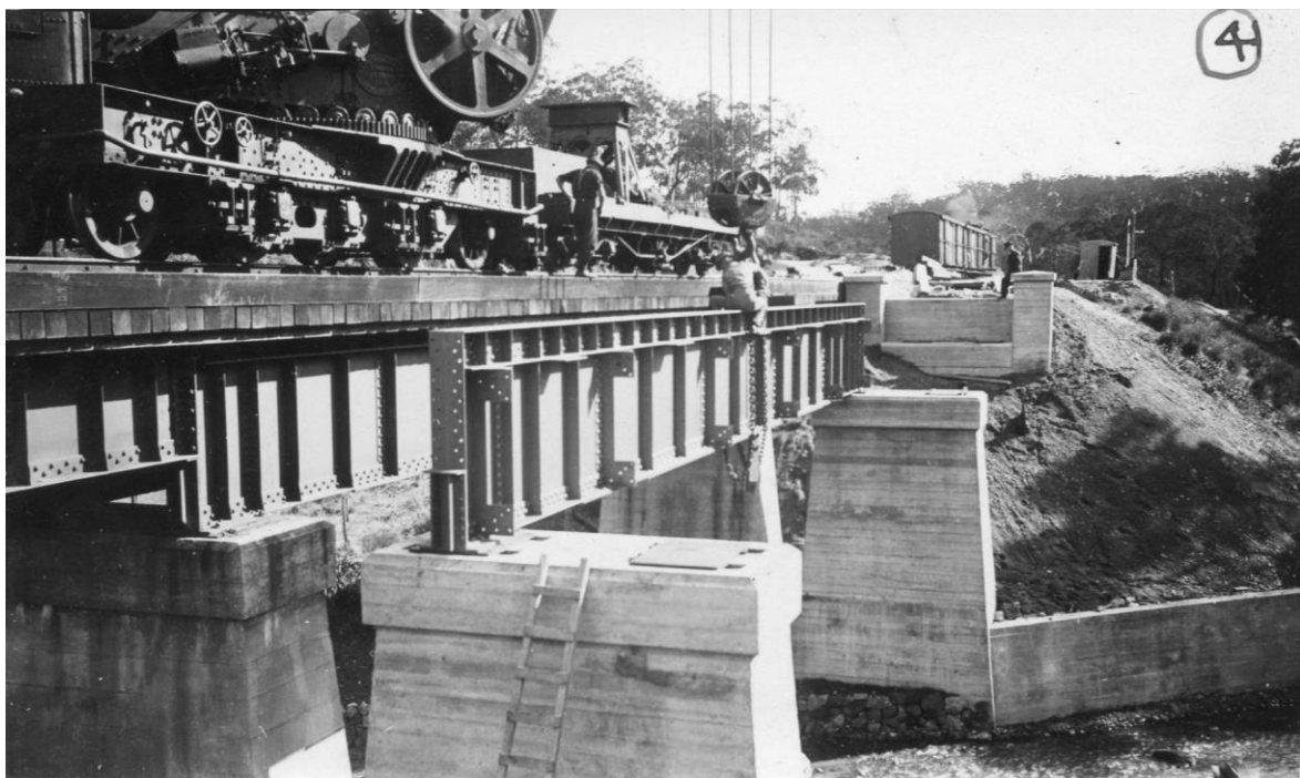
Construction of a steel girder bridge on the Eastern Railway through the John Forrest National Park (date unknown). (Source: Rail Heritage WA, P01431)
