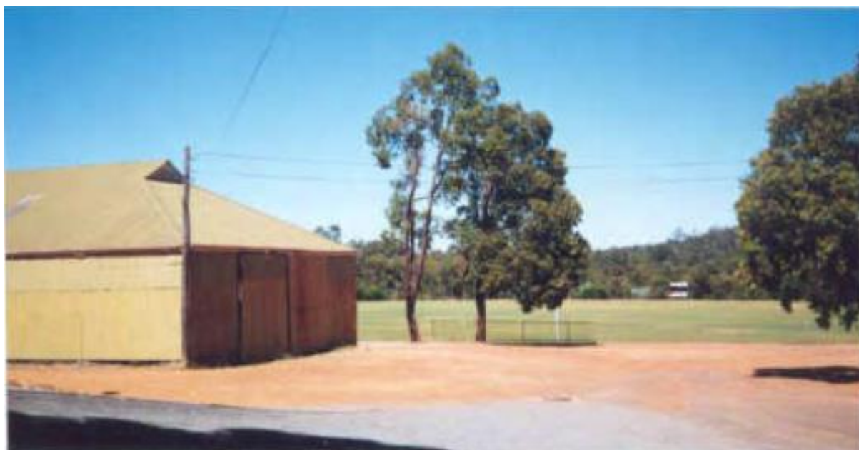
North-east elevation, looking west to ground and score-board (January 1996) (Source: Bruce Callow and Associates Pty Ltd)
