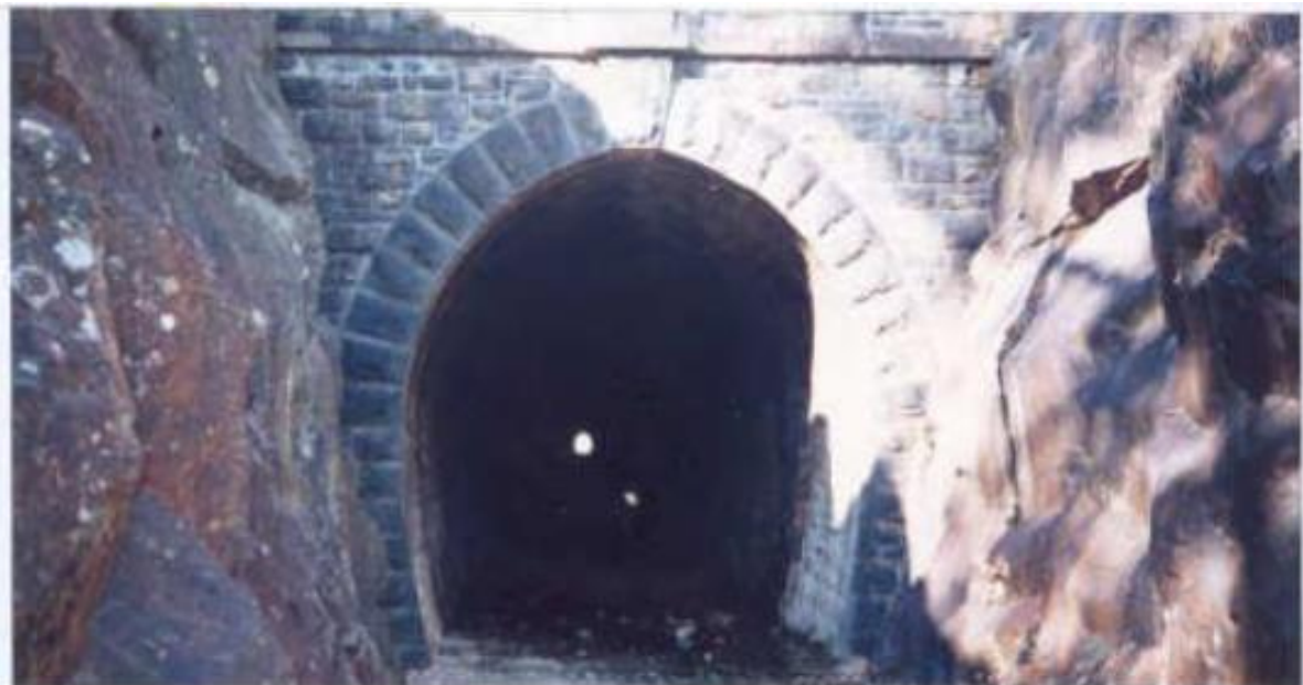
Western entrance of tunnel, November 1995 (Source: Bruce Callow and Associates Pty Ltd)
