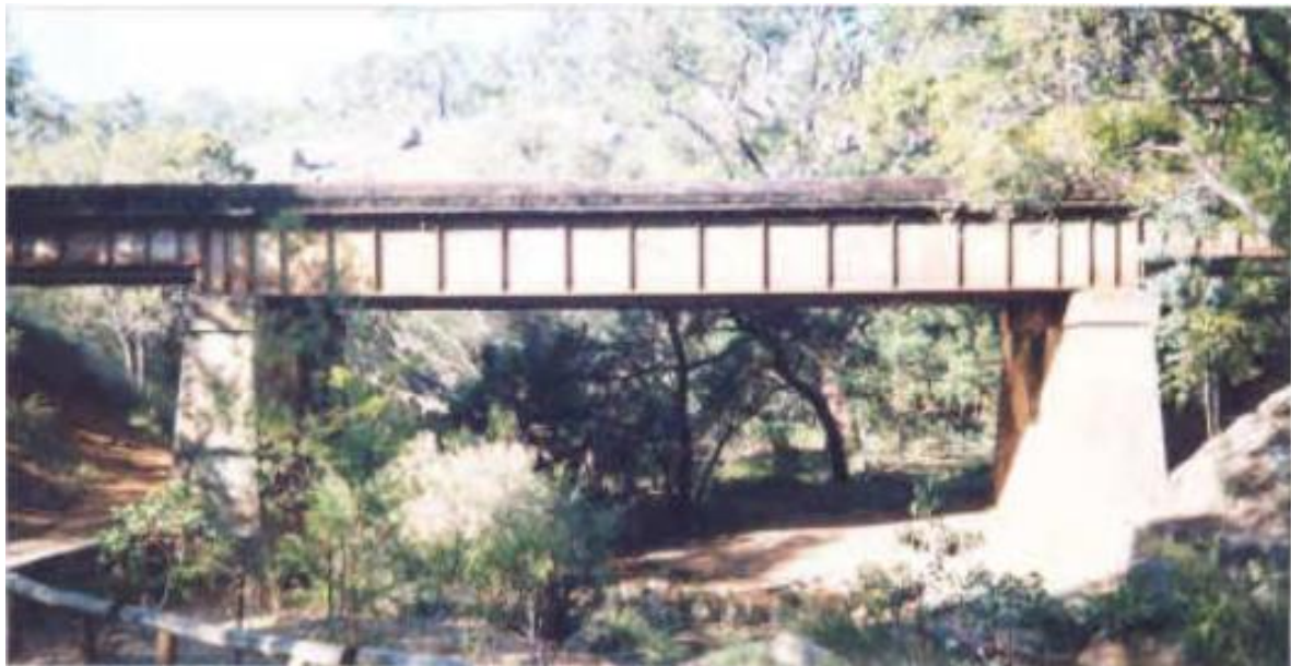
Steel girder bridge in John Forrest National Park, October / November 1995 (Source: Bruce Callow and Associates Pty Ltd)
