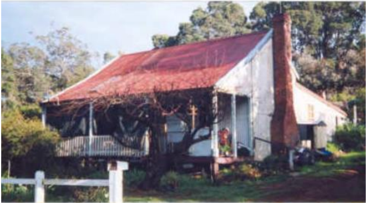
Front, south and east facing elevations, July 1995 (Source: Bruce Callow and Associates Pty Ltd)
