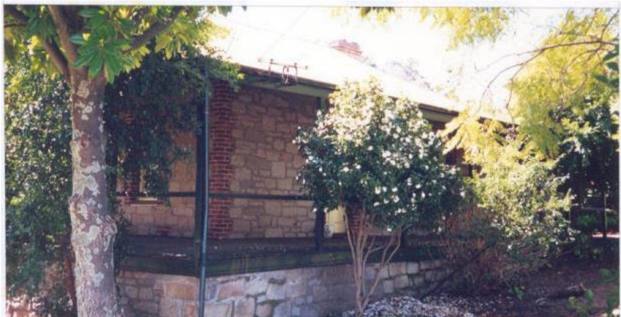
North-west elevation, showing veranda, granite and brick quoins, August 1995 (Source: Bruce Callow and Associates Pty Ltd)
