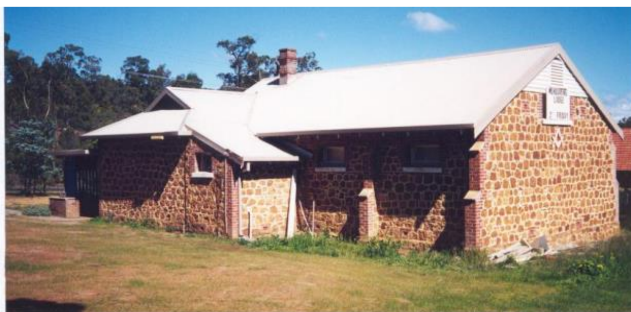
East (side) and North (rear) elevations, August 1995 (Source: Bruce Callow and Associates Pty Ltd)
